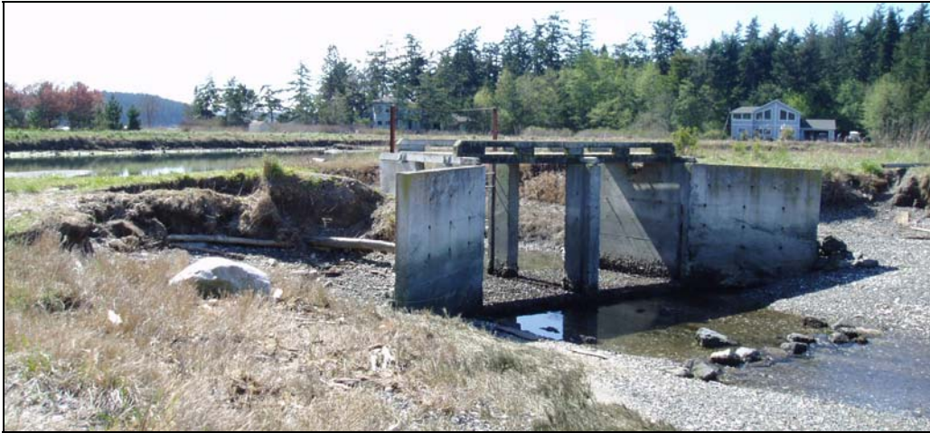
Figure 29. Failed tide gate and constriction at the mouth of Shoal Bay lagoon.
