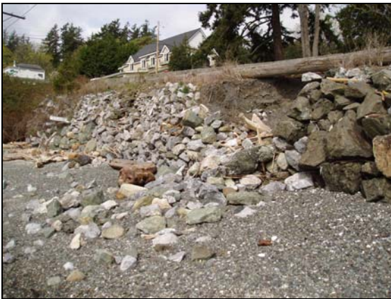
Figure 22. West Sound revetment failure.
